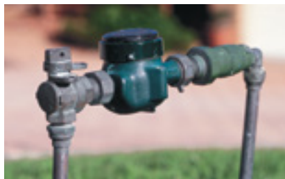
Almost 10,000 aged and faulty meters were replaced by our team in 2017-18
