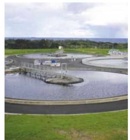
> Burwood Beach wastewater treatment works
