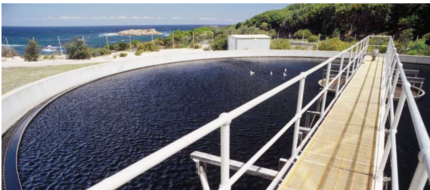
Burwood Beach Wastewater Treatment Works.
